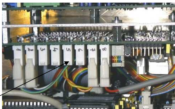
Fig 2: Control relay of the power board
