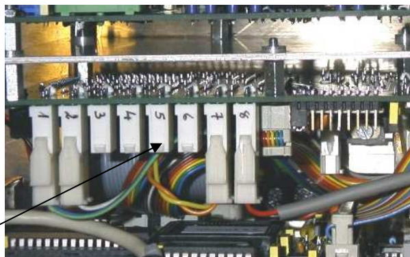
Fig 2: Control relay of the power board
