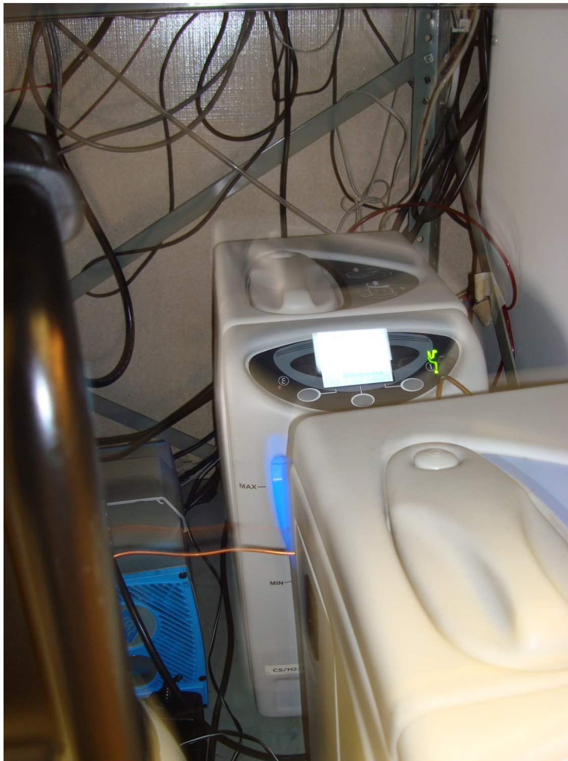
Figure 21: Photograph showing the hydrogen generator employed by CAMs measuring VOCs with a flame ionisation detector.
